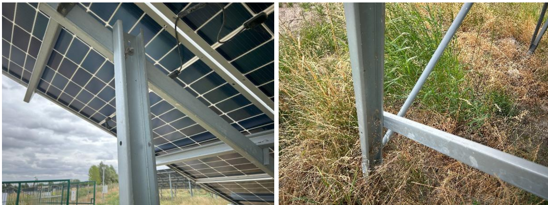
Plate 12-15 Indicative thin racking system driven into ground
